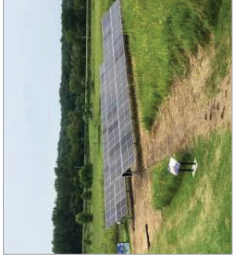
Freestanding solar array at Hurstville Interpretive Center. Photo Credit: Jackson County Energy District website
