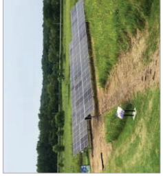
Freestanding solar array at Hurstville Interpretive Center. Photo Credit: Jackson County Energy District website
